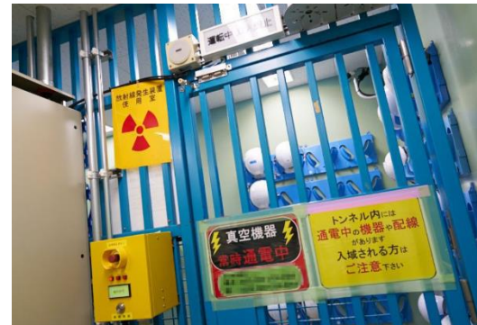
Radiation Control Gate
